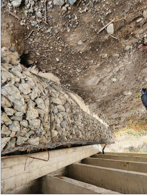
VIEW OF DAMAGED GABION FROM NORTH ABUTMENT (LOOKING NORTH)
